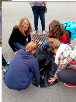
Carter High students install a storm drain insert for the collection of parking lot debris
