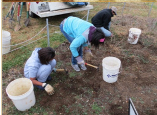
Top two pictures above: Powell Middle School students work with AmeriCorps member to apply erosion control matting on campus hillside
