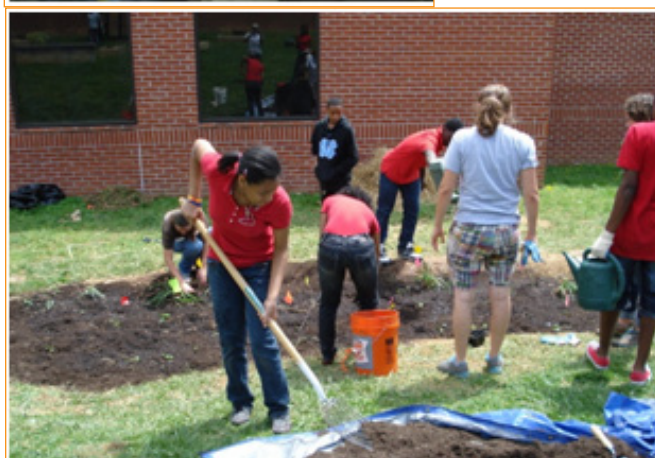
Below: Austin East High School students help to install campus rain garden
