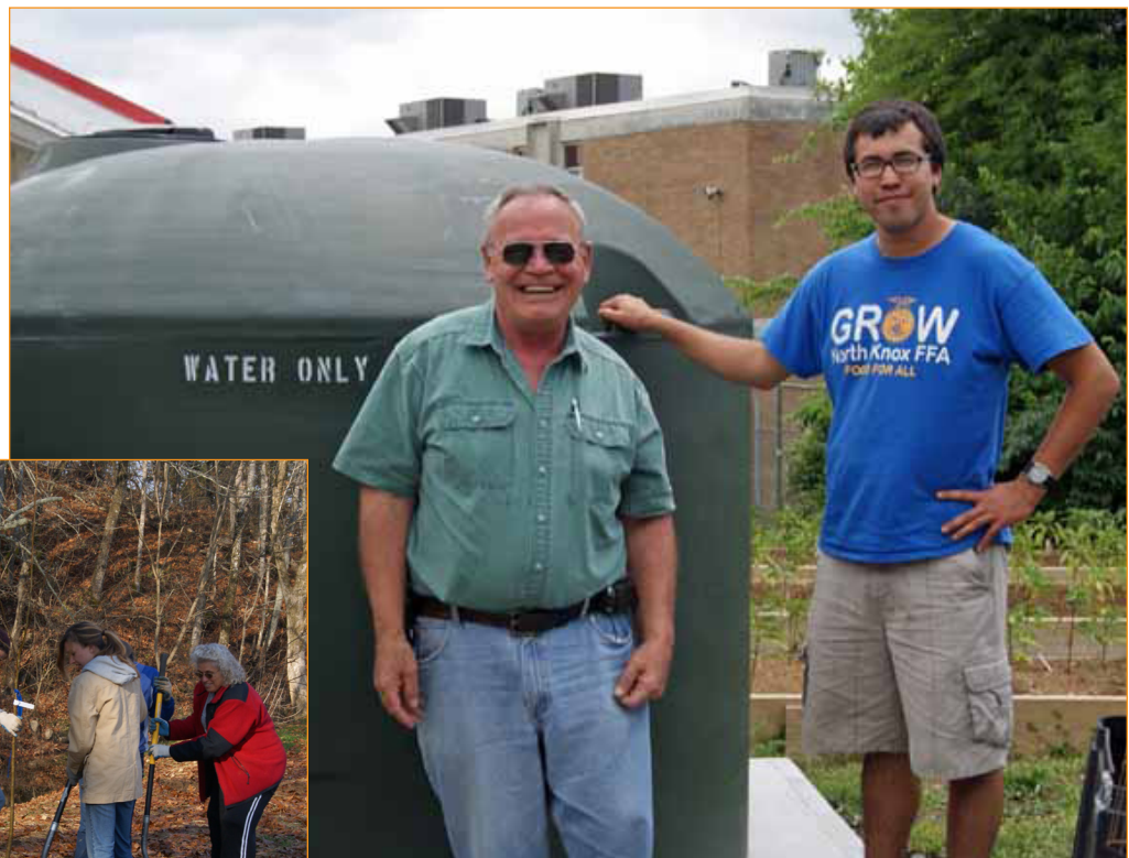
Roy Arthur, TNWRRC, and Elliot Weidow, AmeriCorp Team member in the Adopt-A-Watershed program coordinated by TNWRRC, stand by the newly installed cistern at Halls High School
