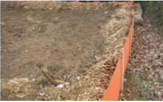
The top three photos demonstrate how silt fences and ground cover can prevent erosion during the construction process. Photo Credit: TNWRRC
