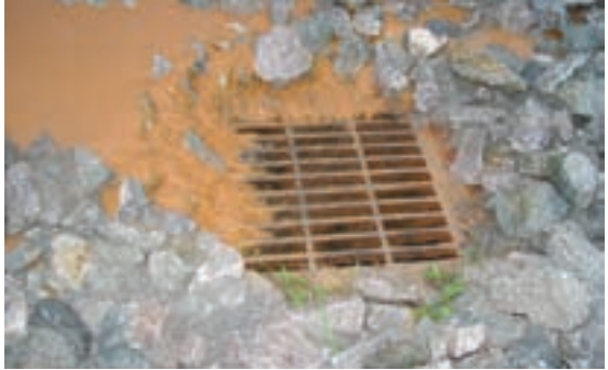
The top three photos depict sediment-laden stormwater runoff, evidence of land disturbance without erosion-control practices. The bottom photo shows one engineered method for keeping soil in place and sediment out of the water. Photo credit: TNWRRC
